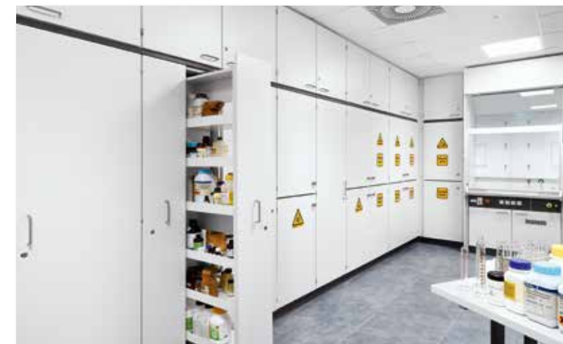
Cabinets integrated into the extraction system and used to store chemicals.
