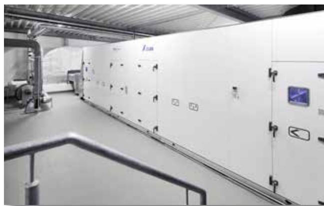
The X-CUBE AHU heats and cools the rooms in the new building.
