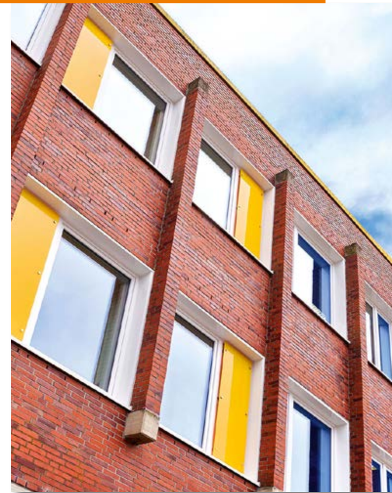
Paul-Spiegel-Berufskolleg vocational college in Warendorf, Germany: narrow window elements have been replaced with opaque elements for air distribution.
