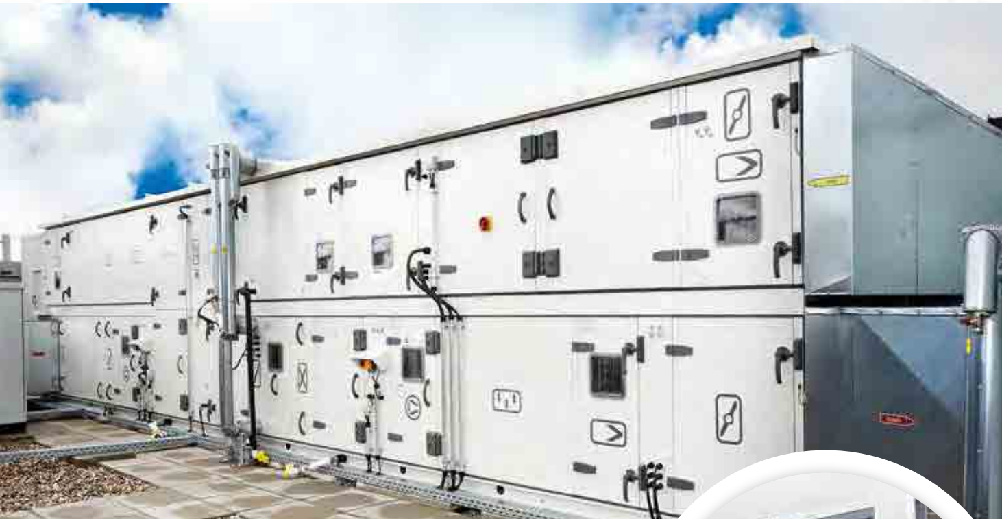
TROX X-CUBE air handling unit on the roof of GERBER.
